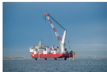
Figure 1: MPI Adventurer installing the anemometry hub off Blyth. Courtesy of Steve McDonald
